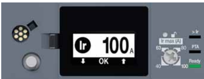
Embedded display Protection settings
